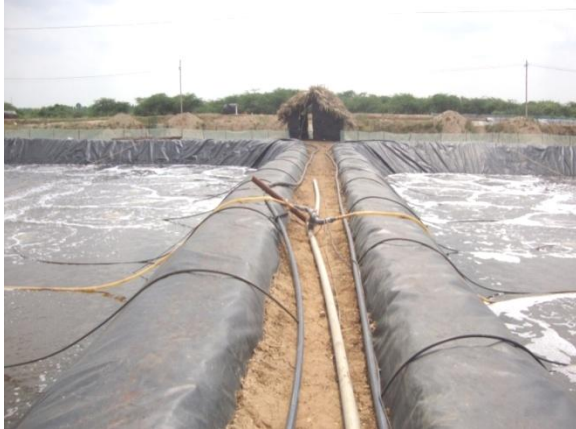
Air distribution by HDPE pipes
